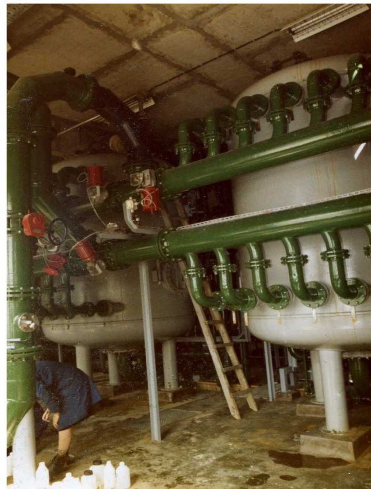
CATION RESIN UP-FLOW COMPACTED BED ION- EXCHANGER - 250 m 3 /h
