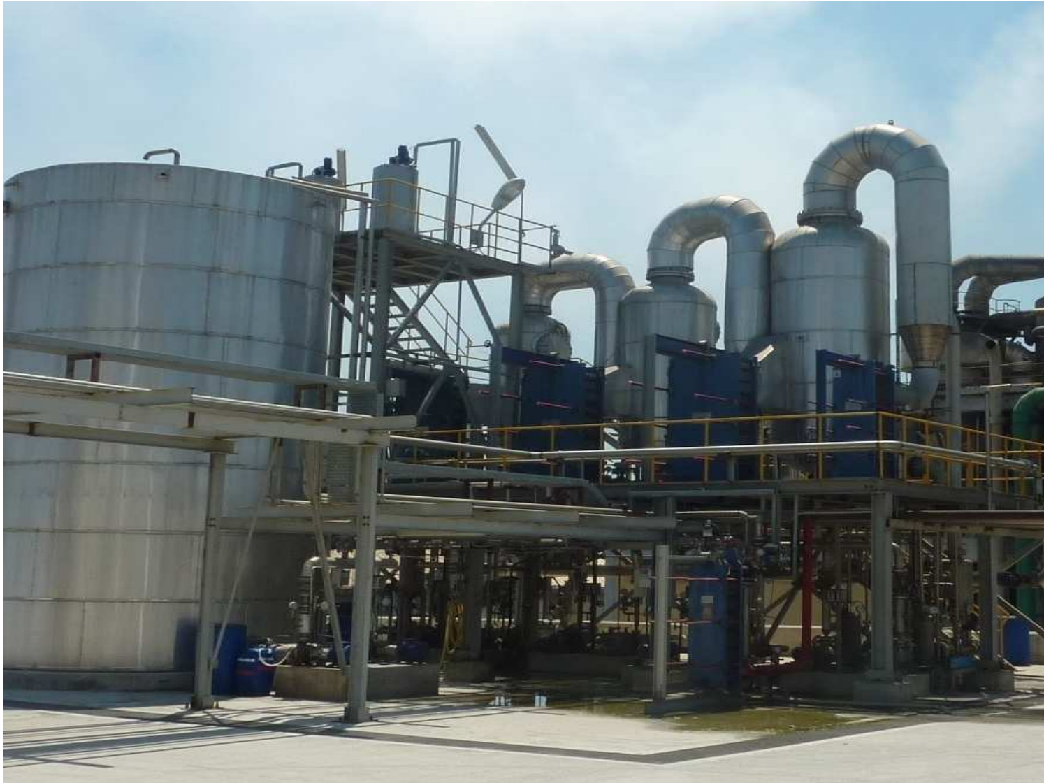
THE NEUTRALISATION AND THE VACUUM EVAPORATION PLANTS 10 m 3 /h
