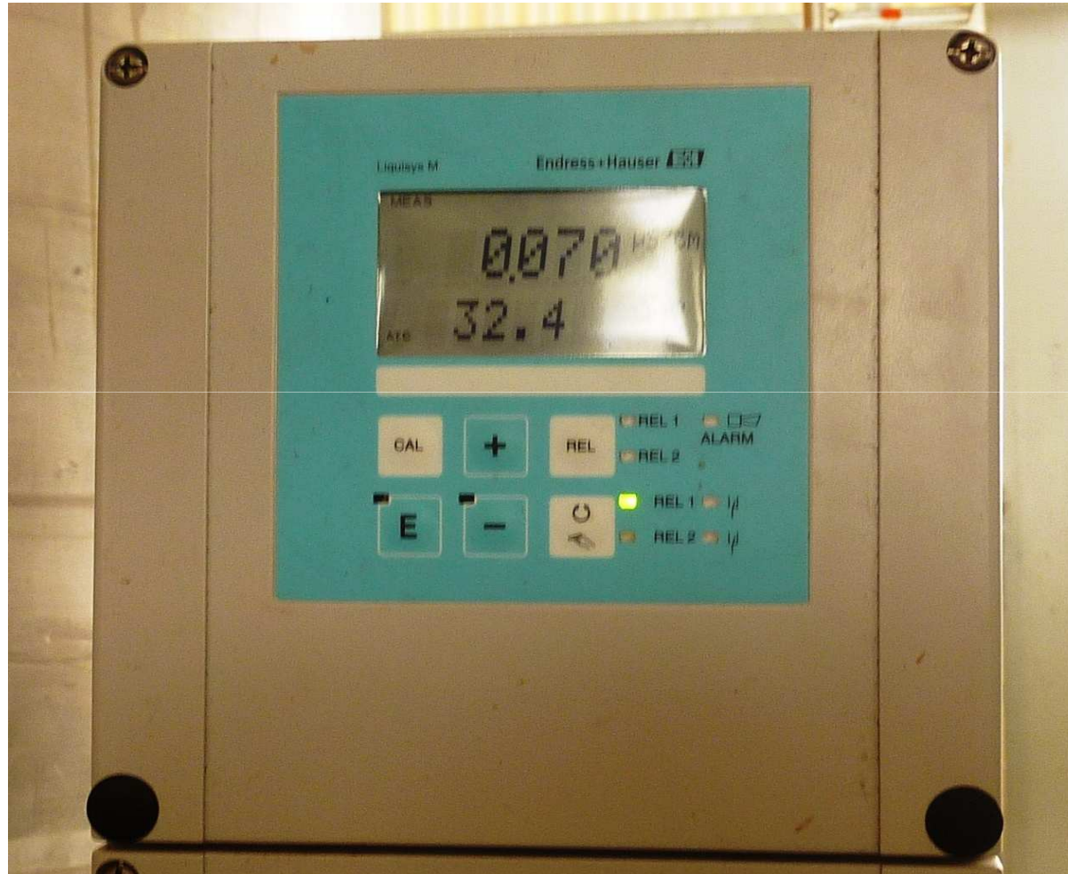
MONITORING OF THE DEMINERALISED WATER CONDUCTIVITY AFTER THE MIXED BED
